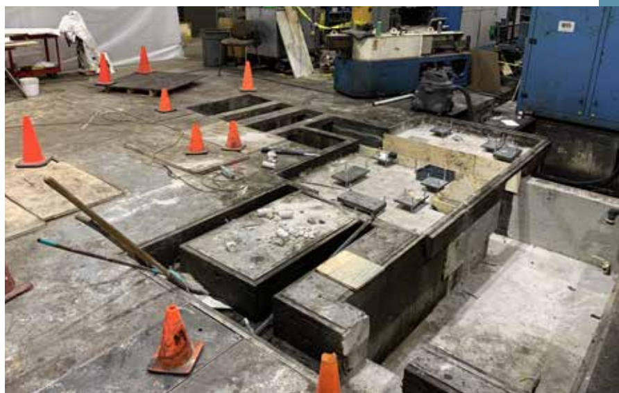
➤ From old to new – step 2: laying the foundation for the new machine.
