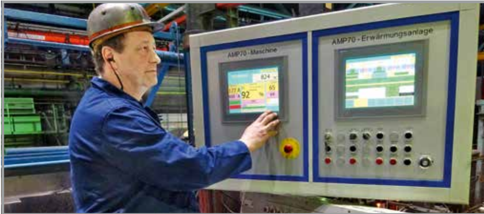
Stefan Görisch checks the current settings for the next production run at the control panel itself.
