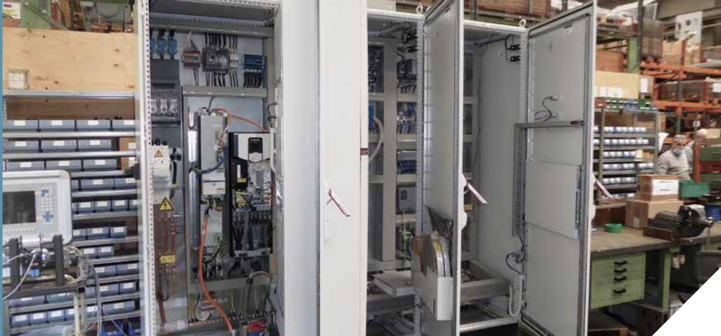
⬆ During the coronavirus pandemic, all of the Hatebur Group's digitalization systems were implemented to perform a remote inspection of electrical cabinets.
