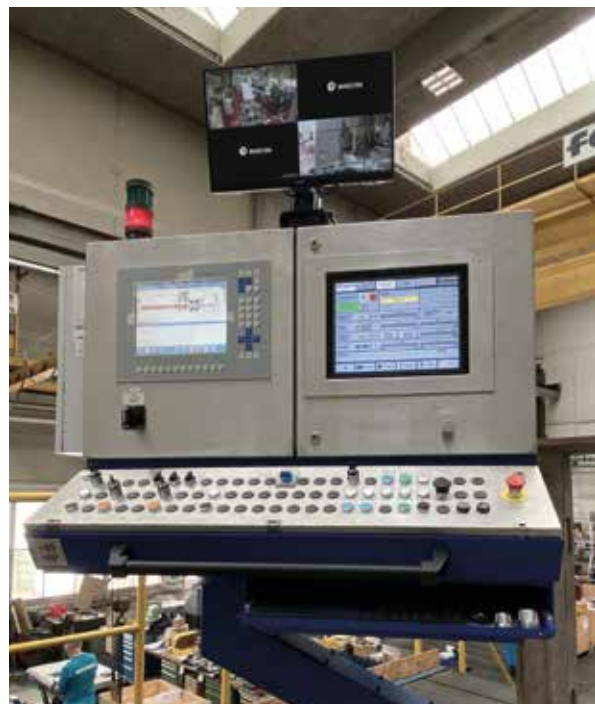
📍 The control desk.
