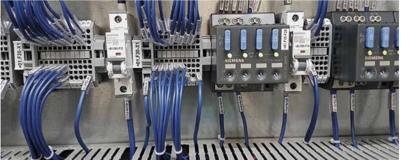
➤ Based on the parts lists, the experts from Carlo Salvi purchase components and cables from Reinach, position the electrical components, wire them and test the finished electrical cabinet in an in-house testing center.
